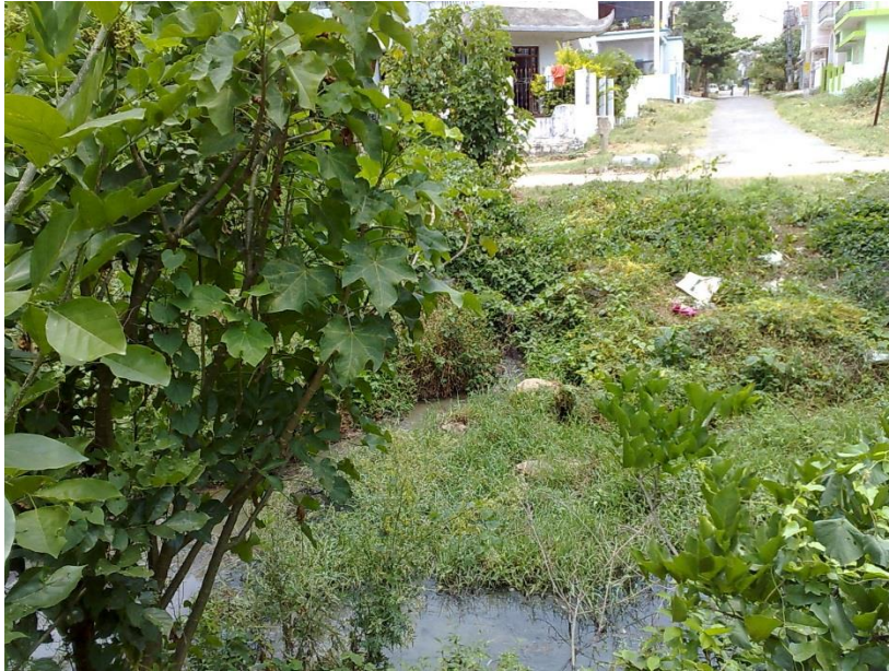
Sewer line bypassed with a pipe laid to connect to the drain at Pathaleeswara nagar
