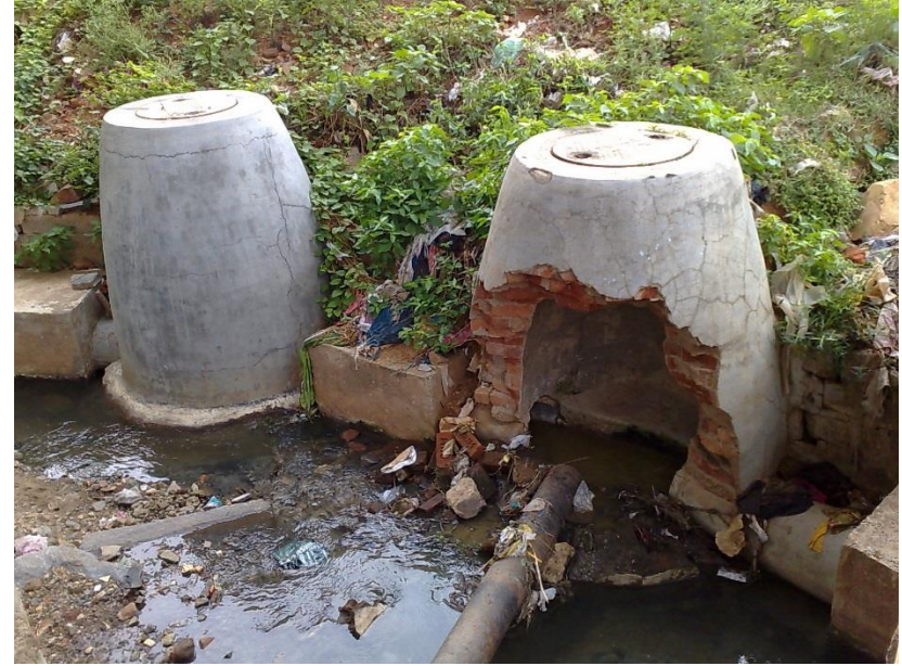
Damaged Manhole to let sewage into SWD at Kumbarkoppal
