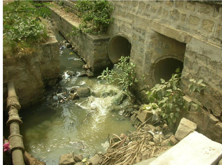
SWD with sewage flow at RMC Market
