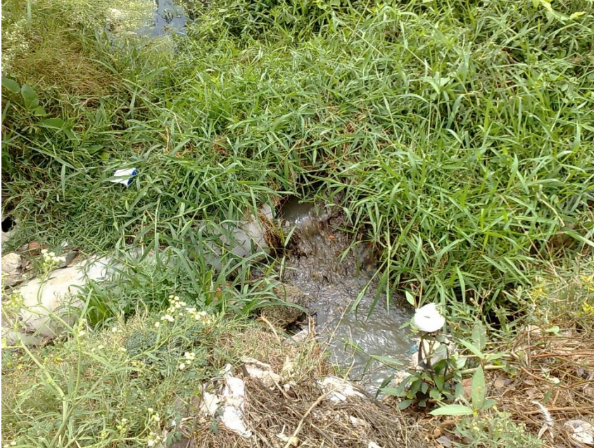
Damaged Sewer at Paduvarahalli
