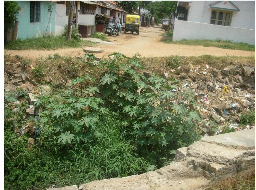
Last MH of the locality after which sewage let into SWD at Bannimantap Ph2
