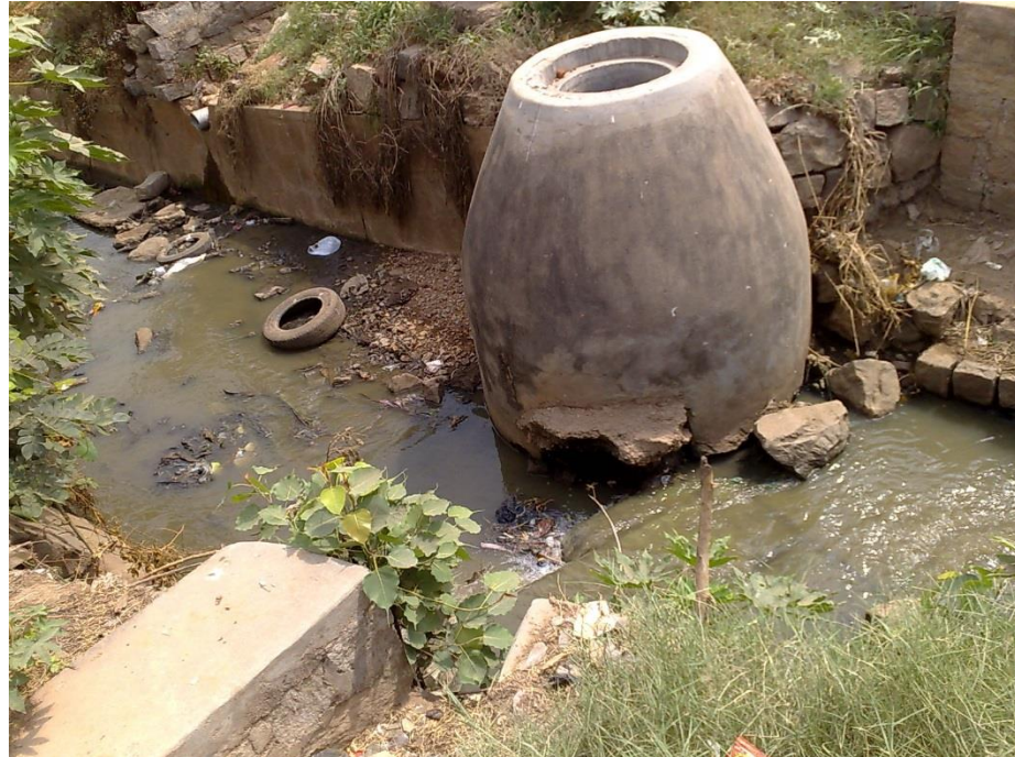
Disturbed MH at Bamboo bazar
