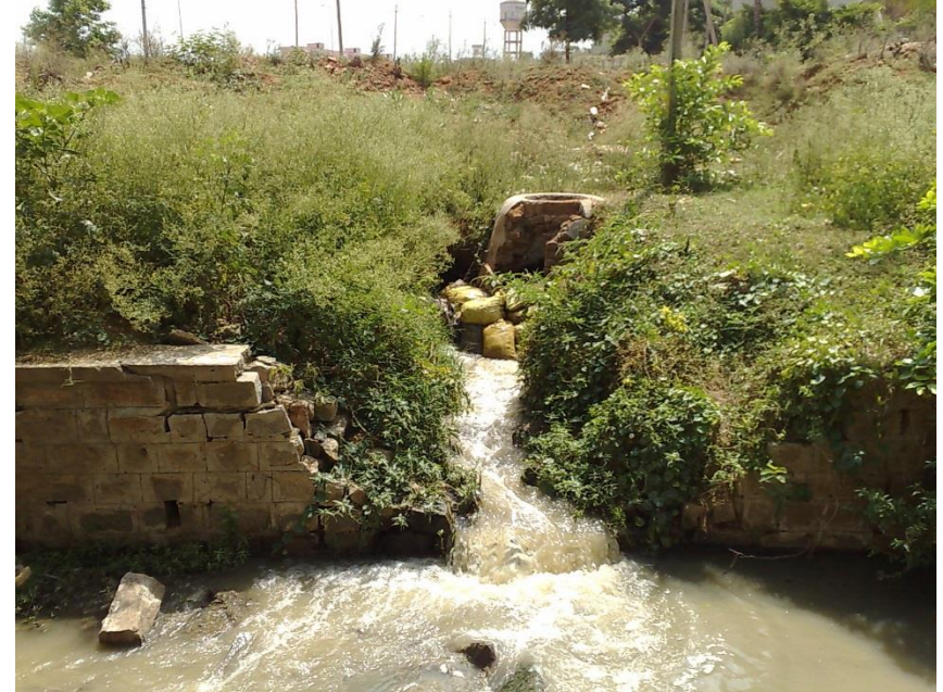
Damaged manhole letting sewage into SWD at Hebbal II- Stage 1
