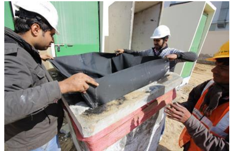
Onsite sanitation units (multiple chambers)
