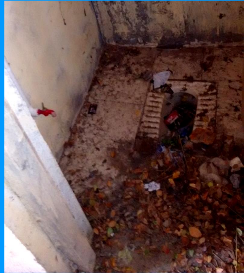
Chocked up toilet due to lack of sanitation staff
