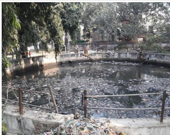
Figure 6: Raw sewage in collection tank with solid waste shows leakage in sewer network
