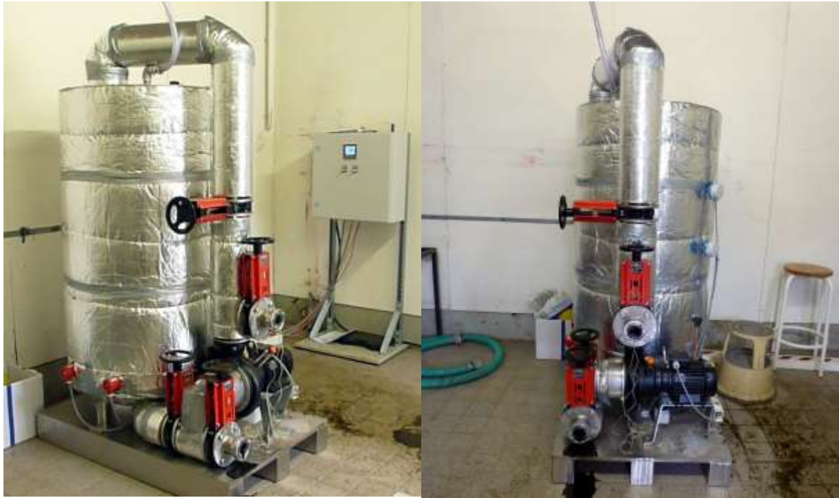
Figure 14: Pasteuriser unit, set-up for laboratory test
