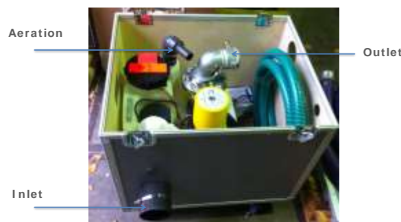
Figure 43: Waste water pump.
