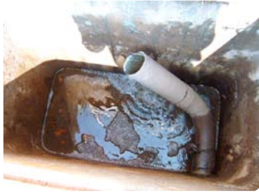
Swivel pipe chamber/ Outlet chamber
