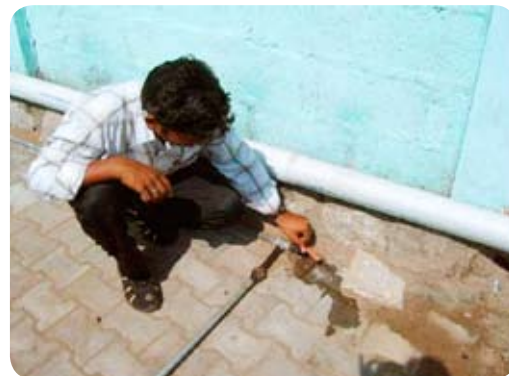
Release of condensed water
