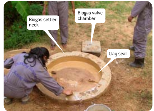
Biogas settler neck chamber
