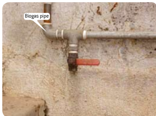
Condensed water release valve
