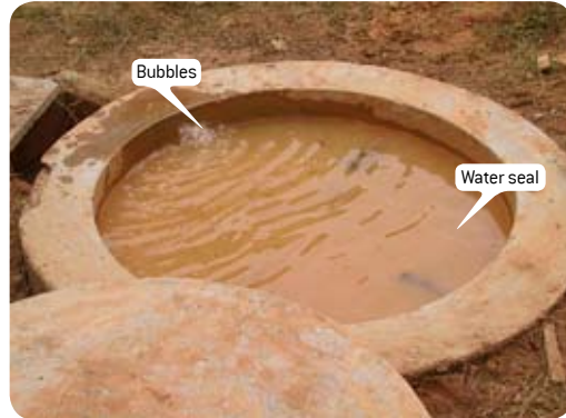
Bubbles indicating gas leakage in the water seal
