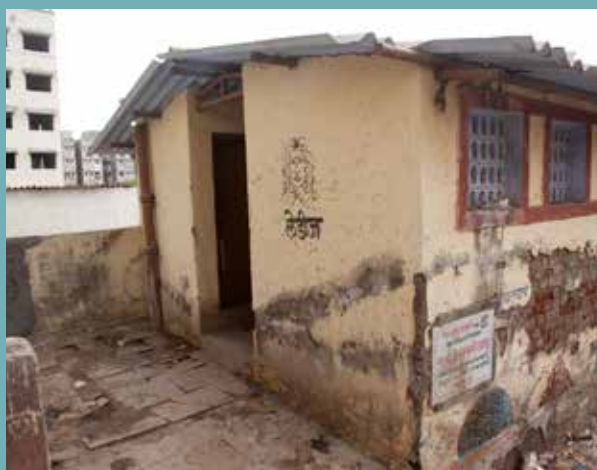
A run-down municipal toilet in a slum in the Vashi Naka locality of Mumbai, India. ©Bill & Melinda Gates Foundation/Prashant Panjari
