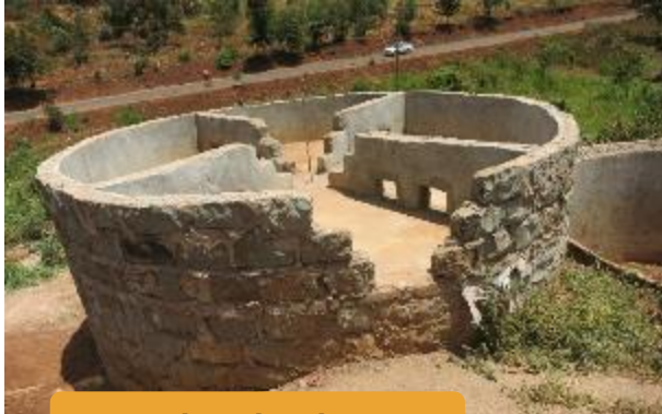
DTF with bio digester
