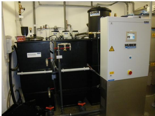
Fig. 8: The completely installed greywater system. On the right is the control cabinet (white).
