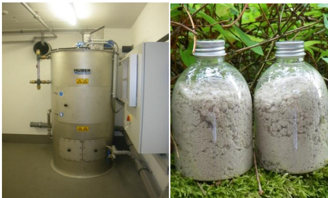
Fig. 6: Left: MAP precipitation reactor manufactured by Huber SE, installed in the basement of house 1. Right: the struvite (MAP) produced.
