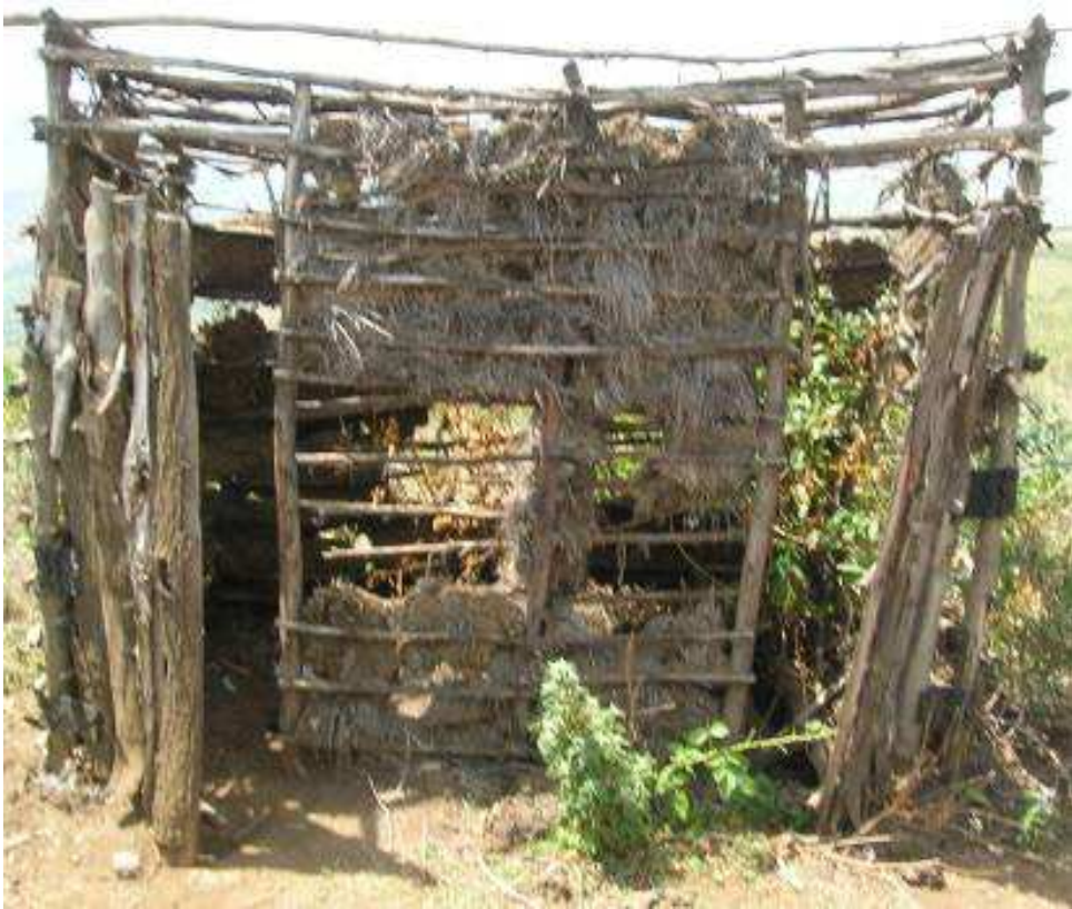
Collapsing pit latrine
