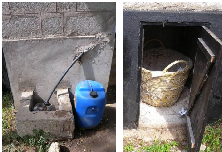
Single vault UDDT in Arusha (Tanzania)
