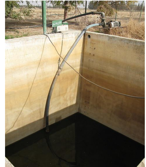
Pump which pumps treated effluent to the fields
