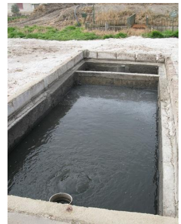
Channel for grit and fat removal
