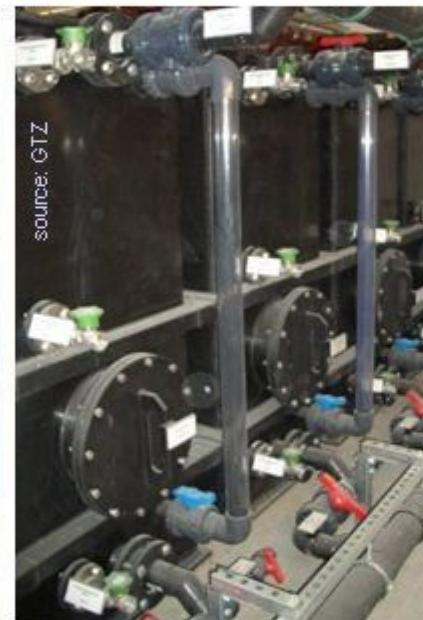
urine storage tanks (4 x 2500 L)
