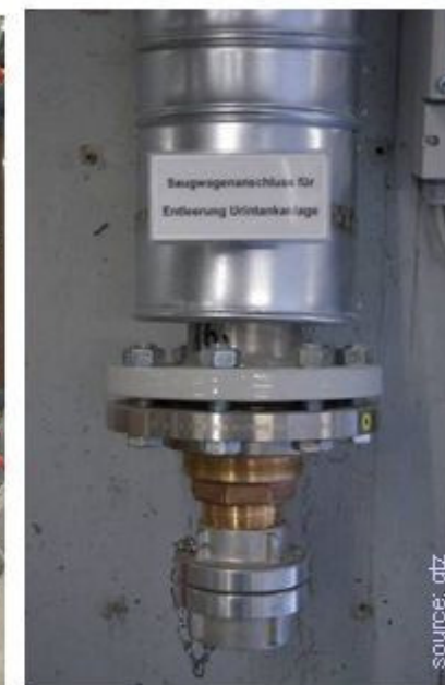
docking station for vacuum tanker
