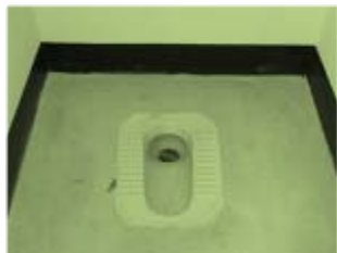
WC usually used in Tanzania (imported). Photo by EEPCO 2006 Approximate cost: Chinese = US $ 6.7, Indian = US $ 7.5
