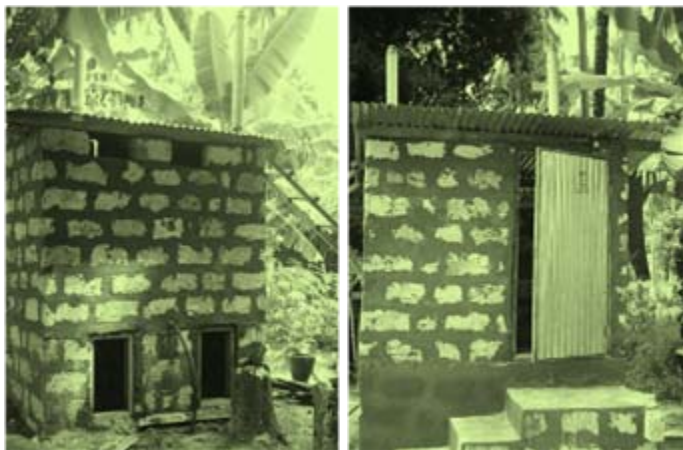
Dry EcoSan toilet under construction for household in Pemba Island. Photos by EEPCO 2006
