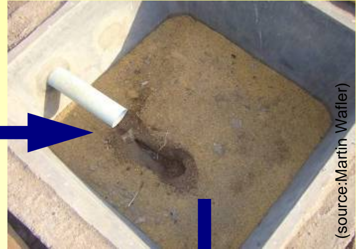
vertical flow filter
