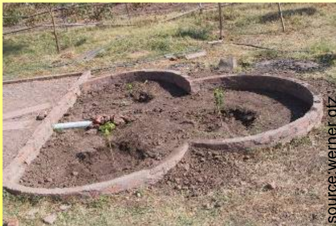
infiltration of anal cleansing water
