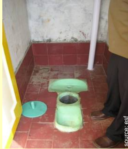
UDD as “emergency toilets“
