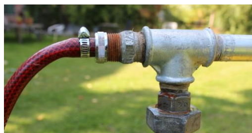
Figure 6: Close up water supply
