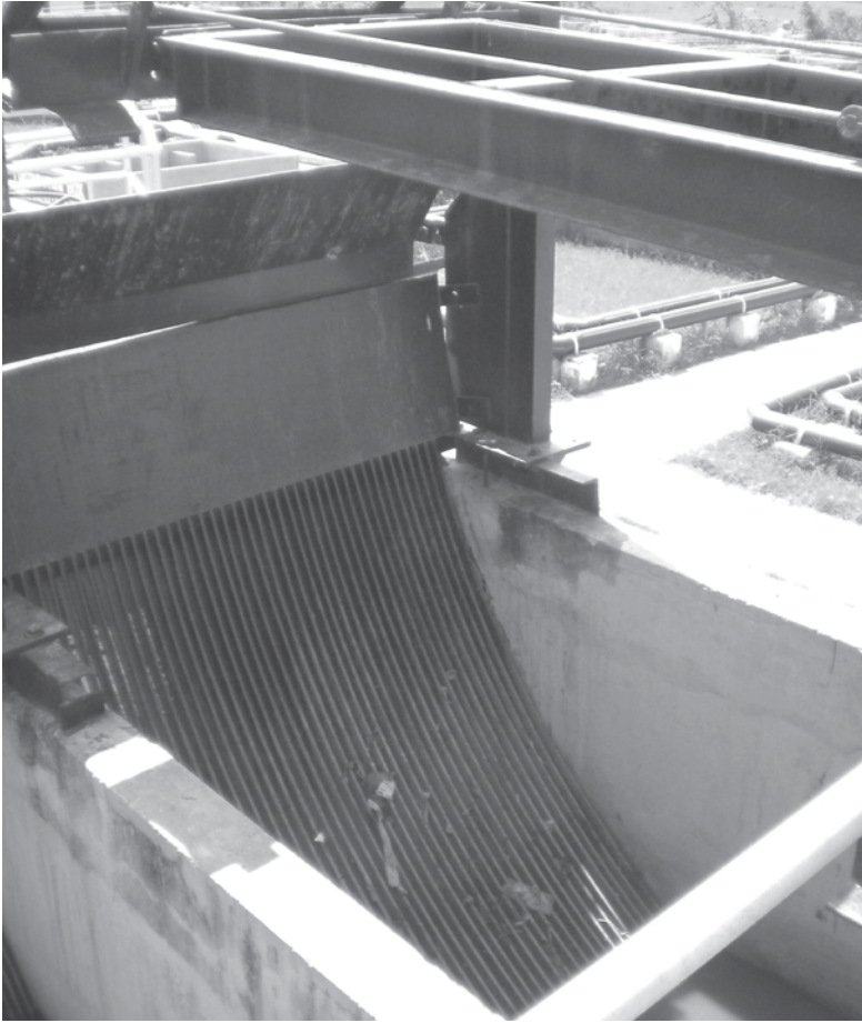
Photo 6.6 Curved screen with rotating raking mechanism
