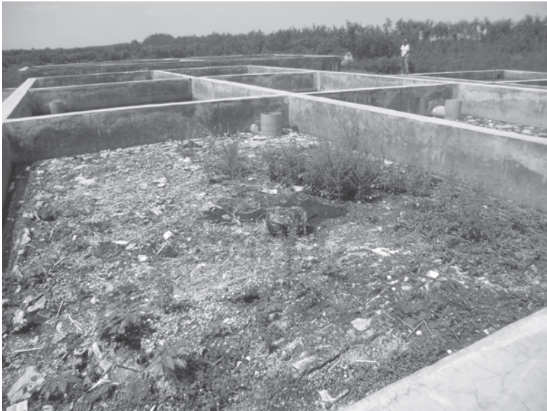
Photo 5.1 Sludge management problems in anaerobic pond, Tegal, Indonesia (note the lack of provision for operator access to the tanks)
