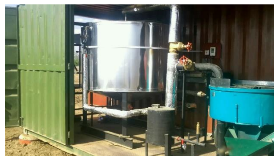
Fig.1: Sanivation dehydration plant (source: Sanivation)
