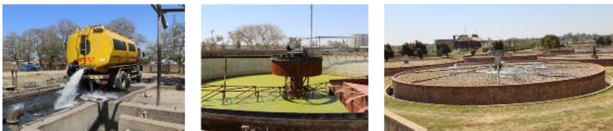
Figure 4: Truck discharging at Manchinchi/dysfunctional clarifier and trickling filter (source: Author)
