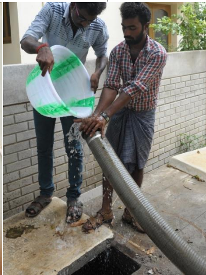
Workers add water to the pipes and the solidified sludge to make the suction process easier. If this doesn't work, they have to enter manually.
