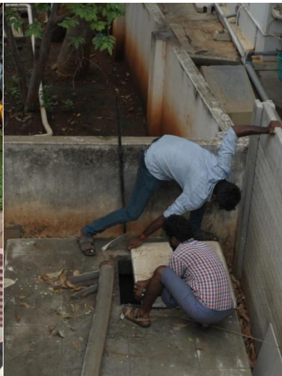
Use rods to open the covers of septic tank. These covers often break inside the tank and workers have to pick them up with their hands.
