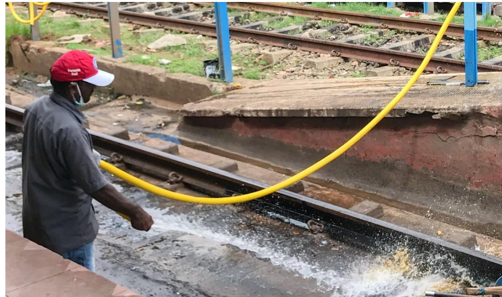
Pick up solid waste from tracks using scooper and put it in a bin; wear gloves and mask. Push excreta into drains using hose pipe (fitted along the tracks).
