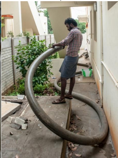
Guide hose inside septic tank, usually without any PPE. Workers occasionally have to enter the tanks when suction doesn't work and/or sludge is solidified.
