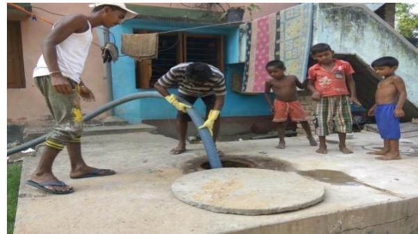
Figure 1: Emptying of a septic tank (Source: Anil/CSE, 2016)
