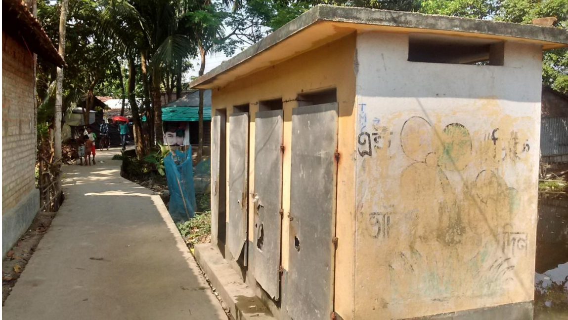
Figure 18: Community toilet in slum (Source: Anil/CSE, 2016)
