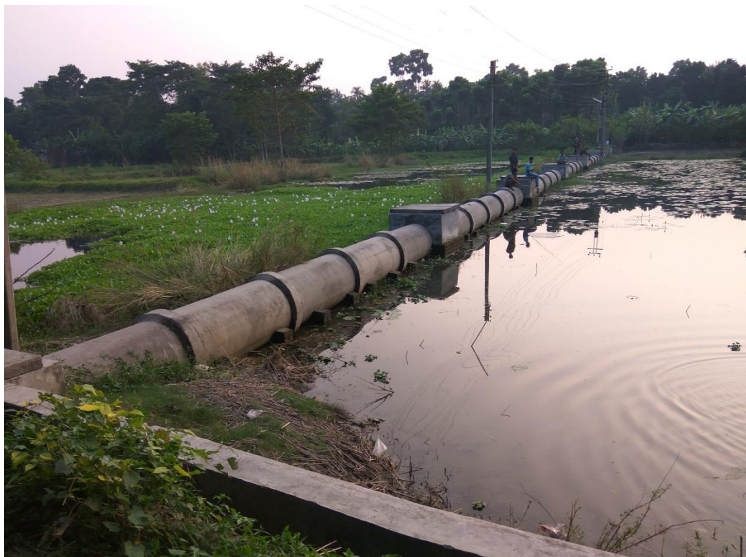
Figure 21: Drain carrying waste water (Source: Anil/CSE, 2016)
