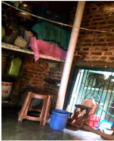
Figure 2: Vent pipe connected to septic tank (Source: Anil/CSE, 2016)
