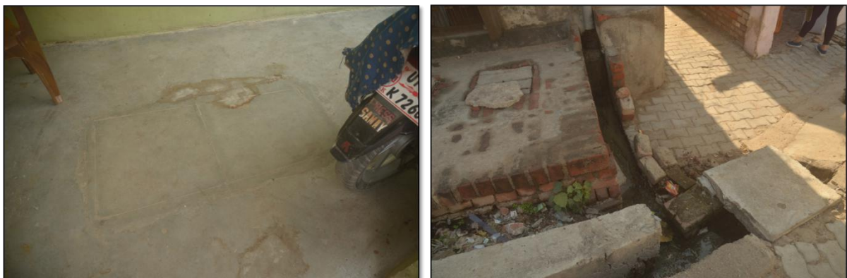
Figure 2: Containment system and its outlet (Source: Amrita/CSE, 2016)
