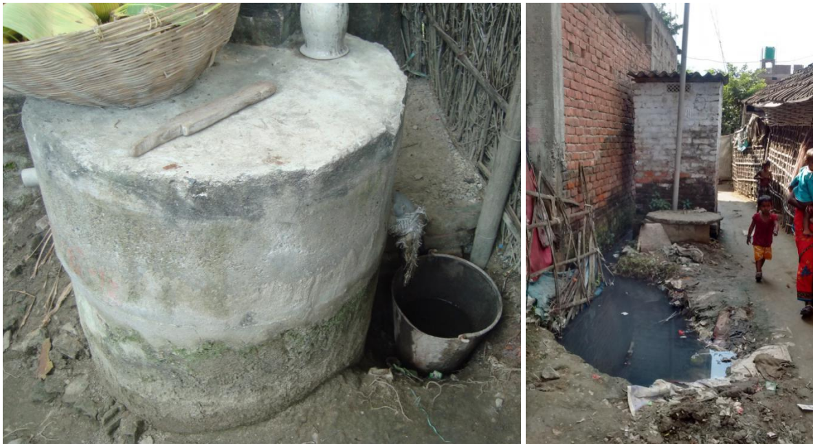
Figure 11: A pit system with temporary solution to avoid frequent desludging (Source: Anil/CSE, 2016)
