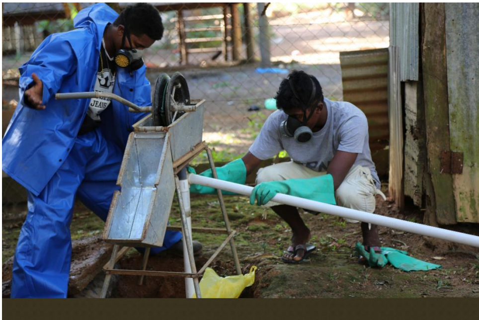
Figure 9: Demonstration of rope pump prototype for extraction of faecal sludge from on-site septic tanks. (WaterAid/Eduardo Rodriguez, 2017)
