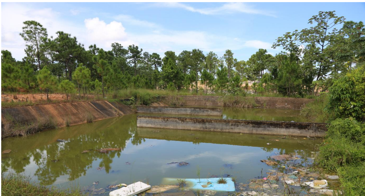
Figure 5 : Inoperative storage pond designed for faecal sludge located at the city garbage dump site. (WaterAid/Eduardo Rodriguez)
