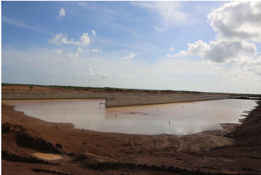
Figure 4: Site of construction of municipal waste water treatment plant, Lamlaya, Municipality of Puerto Cabezas (WaterAid, Eduardo Rodriguez, 2018)
