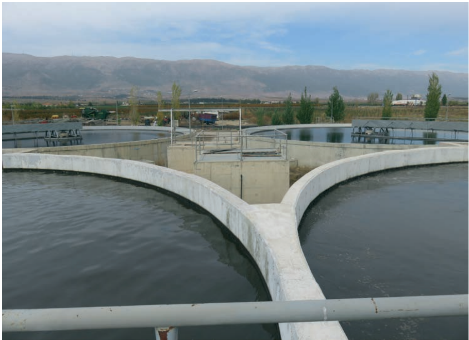
Wastewater treatment station in Lebanon
