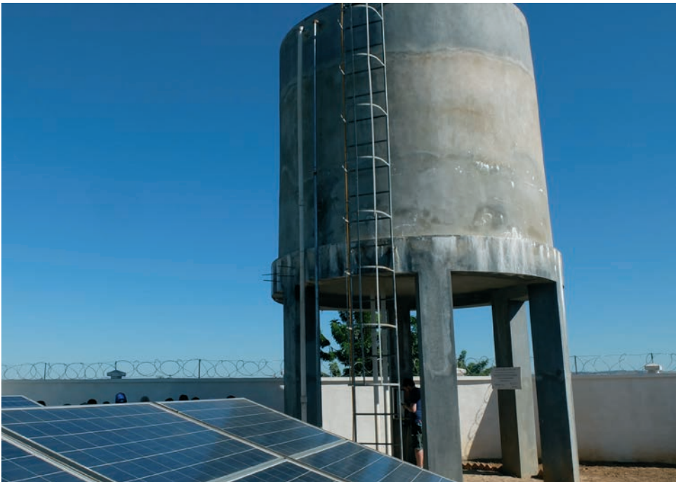
Water storage and solar pumping in Madagascar
