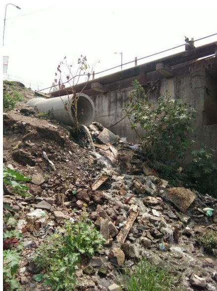
Figure 1: Wastewater from the closed drainage opening to water body (Source: Mrunal/ESF,2018)
