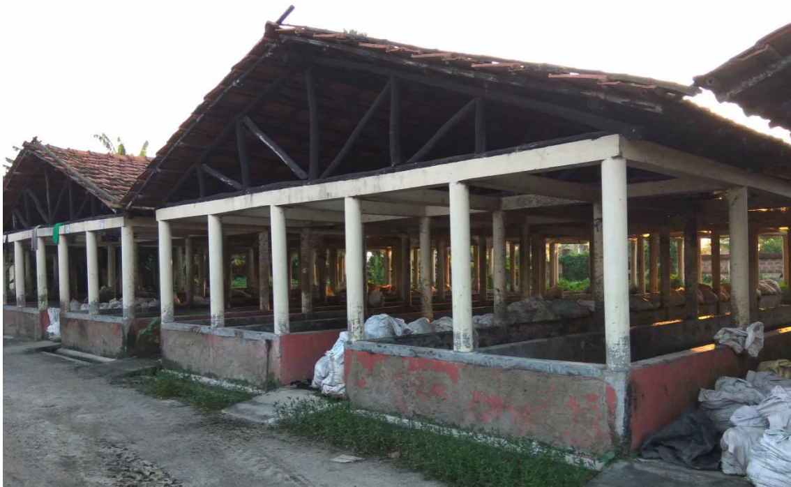
Figure 25: Sludge drying facility at FSTP (Source: Anil/CSE, 2016)
