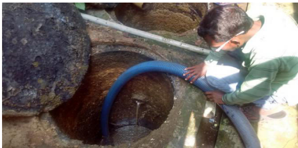
Figure 1: Emptying of a twin-pit latrine (Source: Anil/CSE, 2016)
