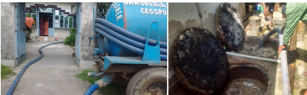
Figure 4: BM vacuum tanker used for emptying septic tank/twin pit system (Source: Anil/CSE, 2016)
