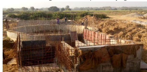
Figure 4: Screens, classifier and equalisation tank of STP under construction at Bijnor (Source: Amrita/CSE 2016)
