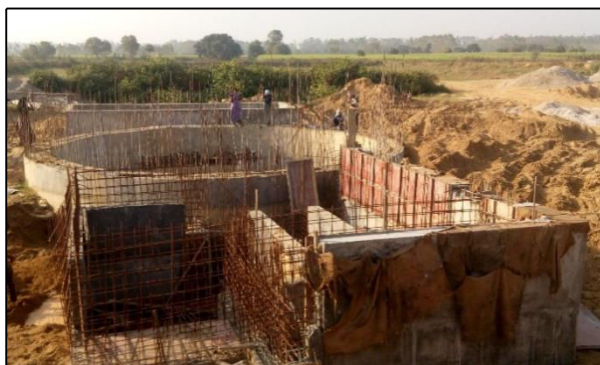
Figure 6: Screens, classifier and equalisation tank of STP under construction at Bijnor (Source: Amrita/CSE 2016)
