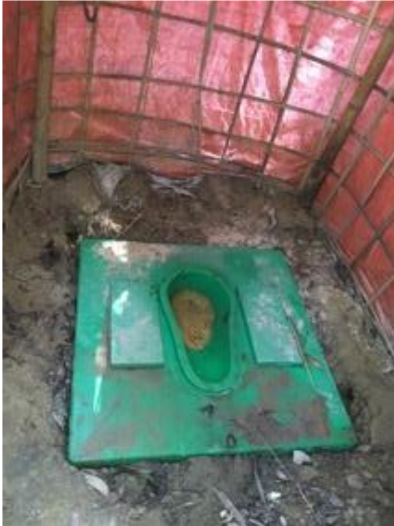
Lack of emptying
