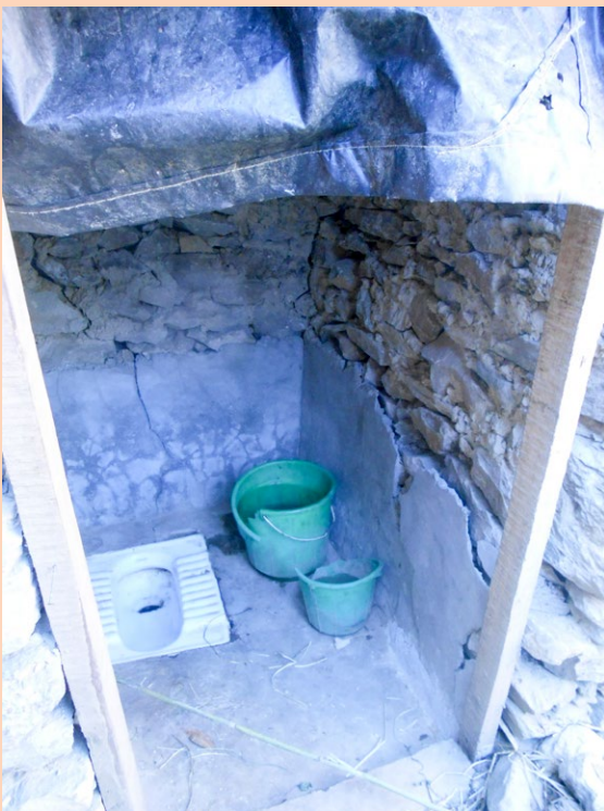
CRACKED LATRINE, RASUWA DISTRICT, NEPAL ©S. HOUSE
