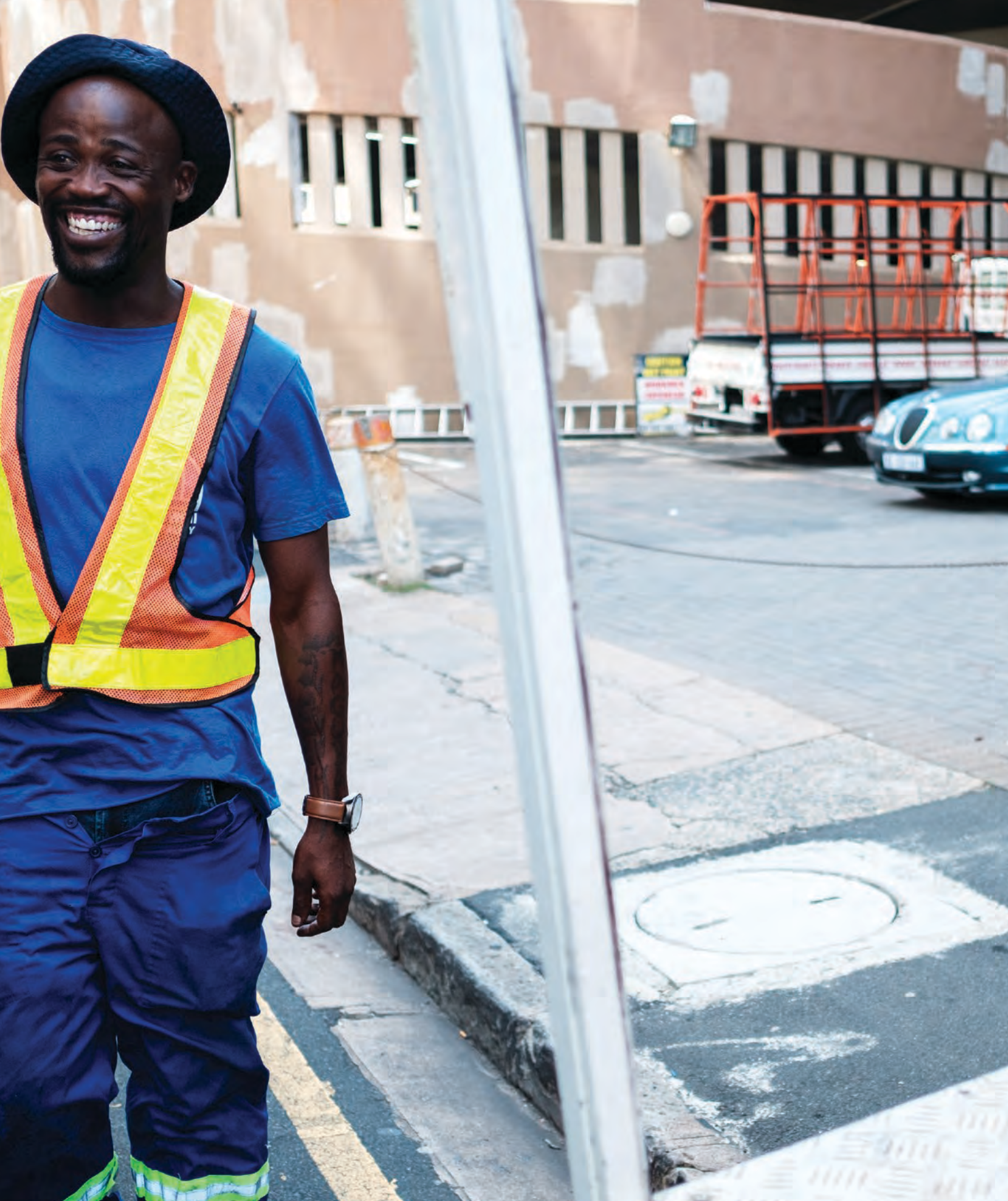
Christopher Magubane (left), 36, and Senzi Dumakude (right), 32, members of an eThekweni Municipality sewage blockage crew at work in Durban. Their team uses flexible rods to clear blockages in pipes leading to the main sewer lines in South Africa, March 2019. © WaterAid / Nyani Quarmyne. Used with permission. Permission required for reuse.
