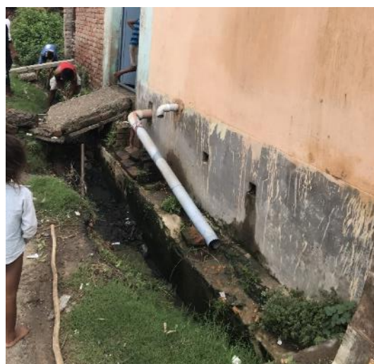
Figure 3: Toilet outlet pipe directly opening into open drain in ward 19 (Harsh/NU/2019).
