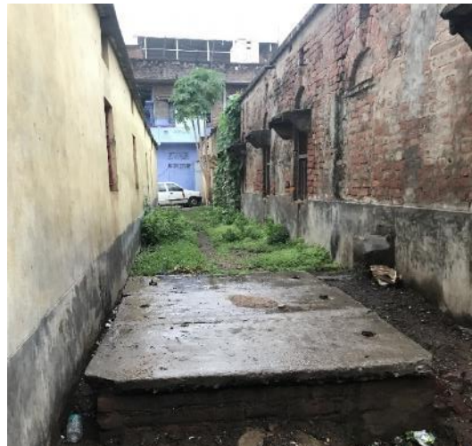
Figure 4: Septic Tank connected to open drain built in between a Lane (Harsh/NU/2019).
