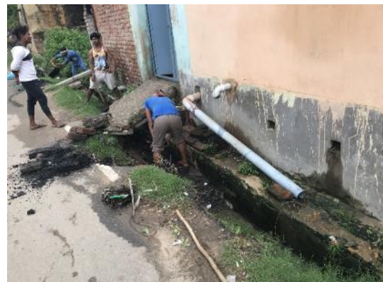
Figure 7: Manual emptiers cleaning the faecal sludge without any PPE (Harsh/NU/2019).
