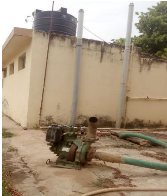
Figure 14: Toilet in Veerayatan premises which gets emptied through Peter Machine (pump set) (source: Gayatri, NU 2019).
