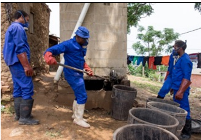
Figure 5 Safe manual emptying by workers contracted by eThekweni Municipality, South Africa. Picture credit: Kathy Eales
