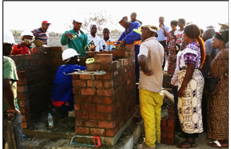
Figure 2 Training builders how to build a good quality toilet – pictured here in Lusaka, Zambia – is an essential step towards providing a workable regulatory framework for non-sewered sanitation and FSM. Picture credit: Mukaku, M. N.
