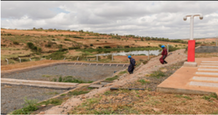
Figure 5 One of Kenya's new decentralised sludge treatment plants. Picture credit: Water Sector Trust Fund
