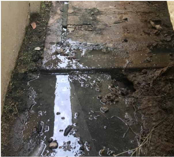
Figure 3 : A damaged household connection with leakage on the road in Zone 13 (Kripa/Eawag/2019).
