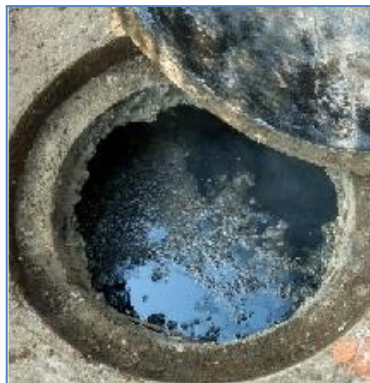
Figure 12: Sewage being discharged into a storm water drain in ward 145 (Kripa/ Eawag/2019).
