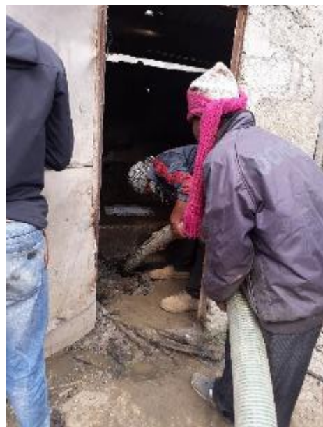
Figure 9: Desludging Labour in action without any protective equipment
