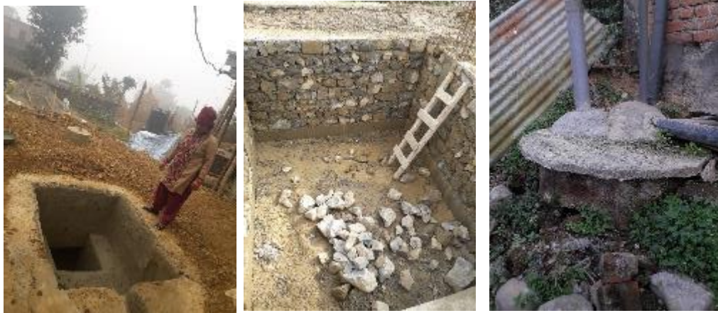
Figure 7: Construction of Anaerobic Biogas Digester, Lined tank with open bottom and semipermeable lined pit with open bottom
