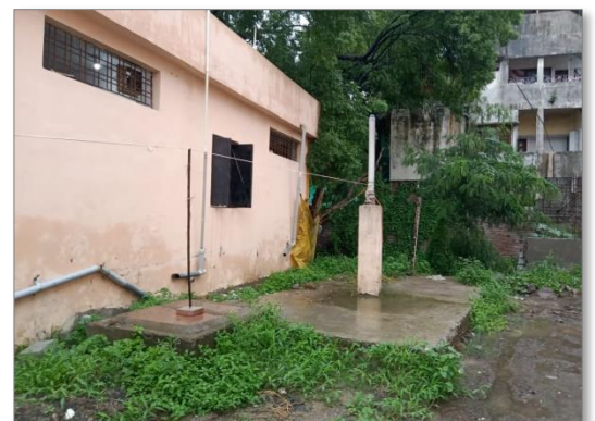
Figure 2: Septic tank of a public toilet located at Collectrate, Moti Tabela
