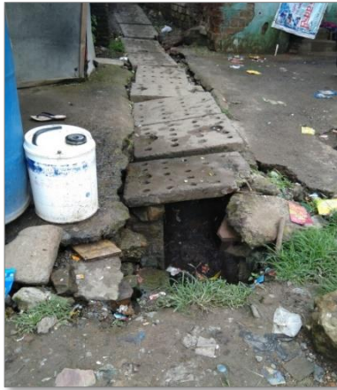
Figure 1: Open drains carrying wastewater in Kabutar Khana
