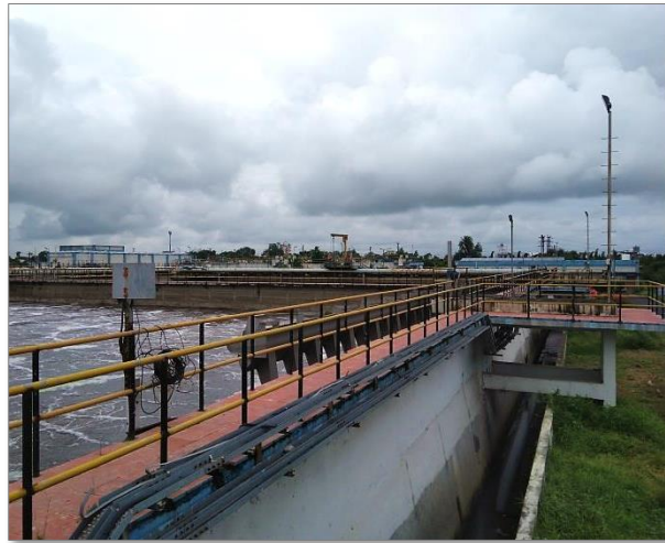
Figure 4: Sequencing Batch Reactors (SBR) for STP of 245 MLD capacity
