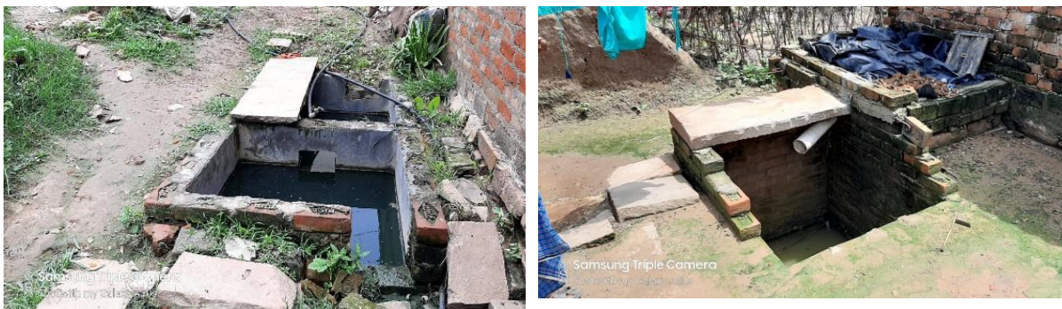
Figure 1: Septic Tank under construction and fully lined tank connected to open drain (Manish/CSE,2020)
