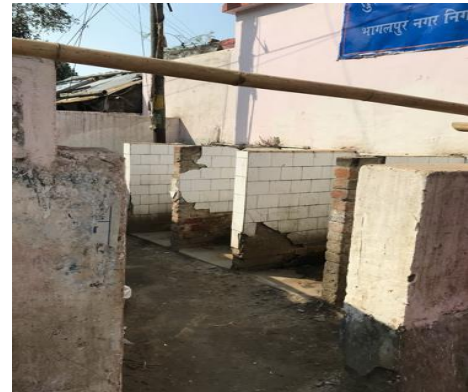
Figure 6: Urinals in of the CT and PT in the commercial area of the city (Source: Harsh/CSE 2020)
