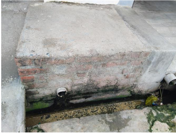
Figure 3: Fully lined tank connected to open drain
