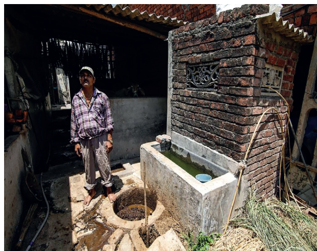
Toilet-linked biogas plant in Valsad district, Gujarat
