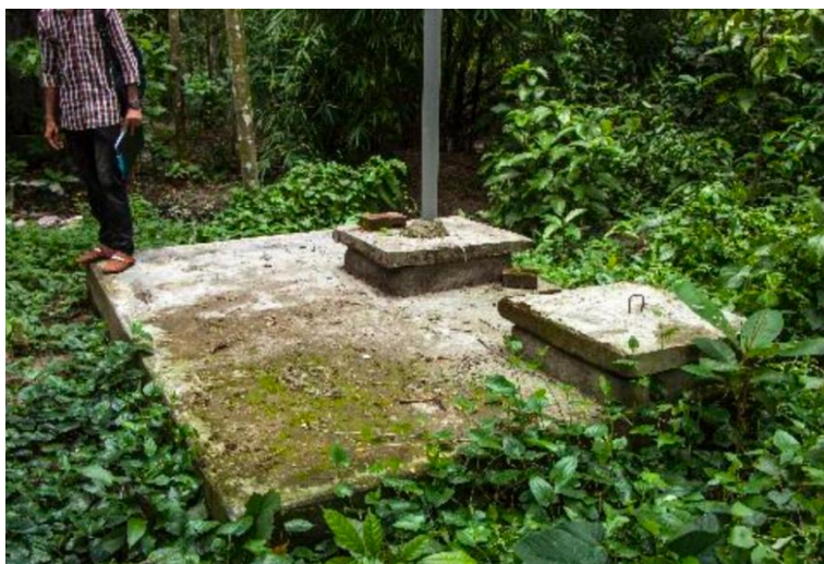
Figure 7: Septic tank in Bhola (Source: UPM 2019).
