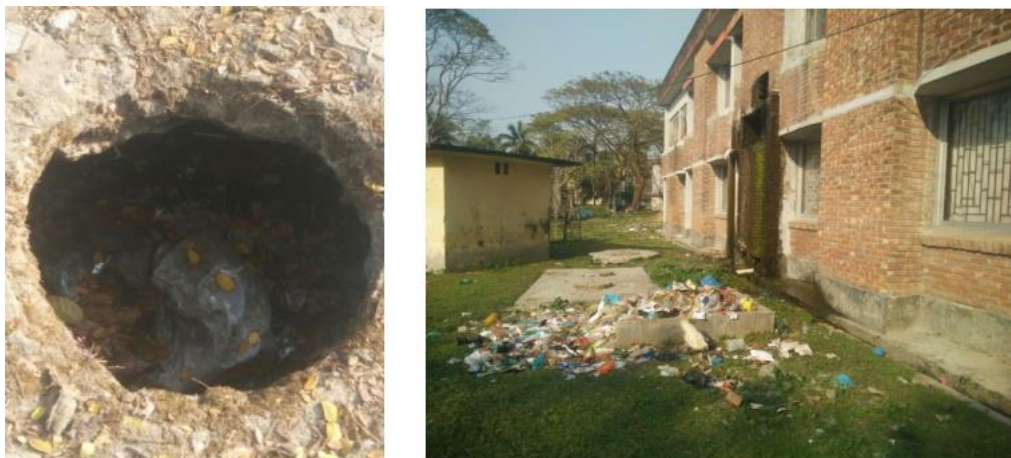
Figure 9: Open septic tank clogged with solid waste and solid waste disposal at the of Bhola public hospital (Source: UPM 2020).
