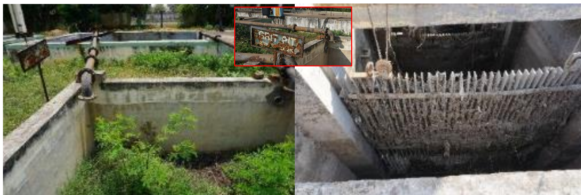
Figure 4.14: Grit Pit and Screening Systems – Not Being Maintained in Anna Stadium
