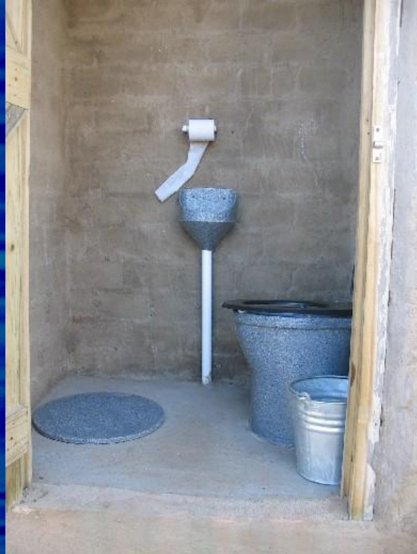
Left: Closed vault Middle: Waterless urinal Right: Plastic UD pedestal and bucket with sand
