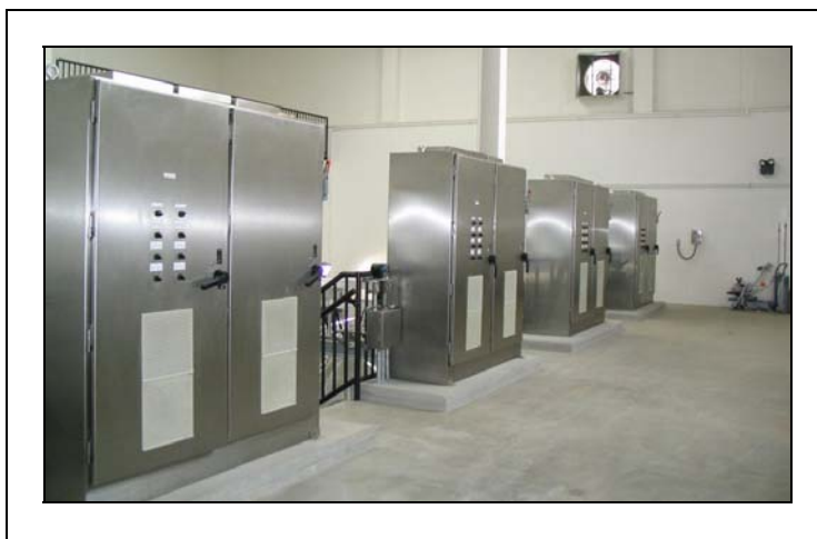
Figure F.14. UV Reactor Electrical Cabinets at the Weber WTP No. 3 (the floor above the UV reactors)
