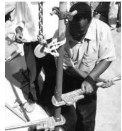
Riser pipe with pipe clamp & attached hook
