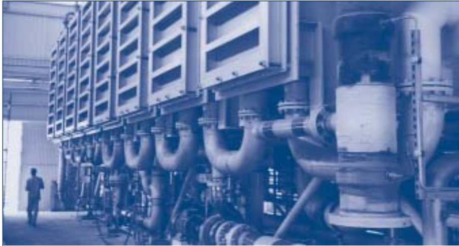
Fig. 18.2. Multi-effect distillation plant with vapour compression (MED +VC) in Mindelo, Cape Verde (capacity: 2400m 3 /day) (photograph by Jan C. Schippers)
