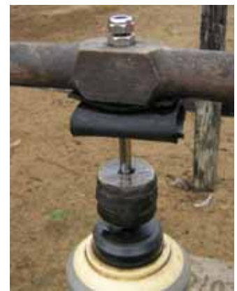
Long pumprod cleverly solved by the community by attaching several rubber discs made from car tyres.
