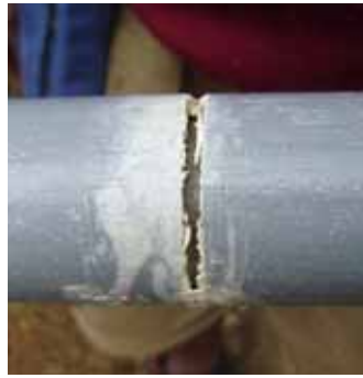
Bad pipe joint
