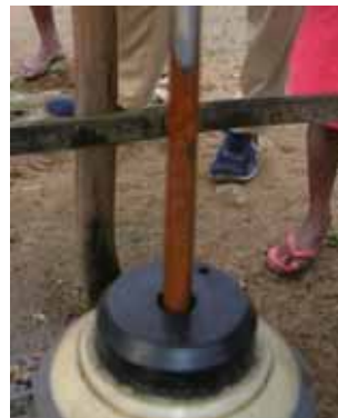
Mahalevona MV 27, red staining on pumprod on inside of pump housing
