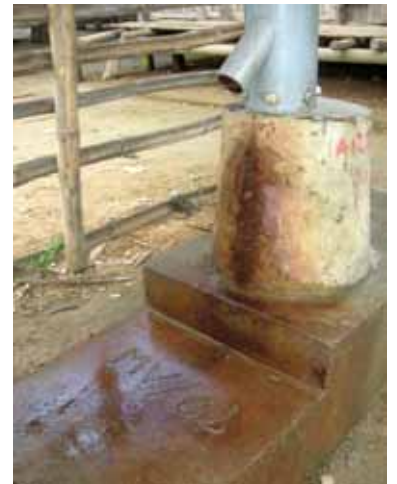
Mahalevona MV 02, pump stand with red marks, (iron staining)
