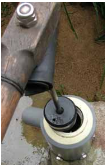
Antoraka AT 02, eccentricity (sign of a bent rising main)
