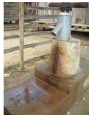
Red staining (iron)
