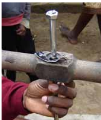
Andranofotsy AF 13, broken pumprod
