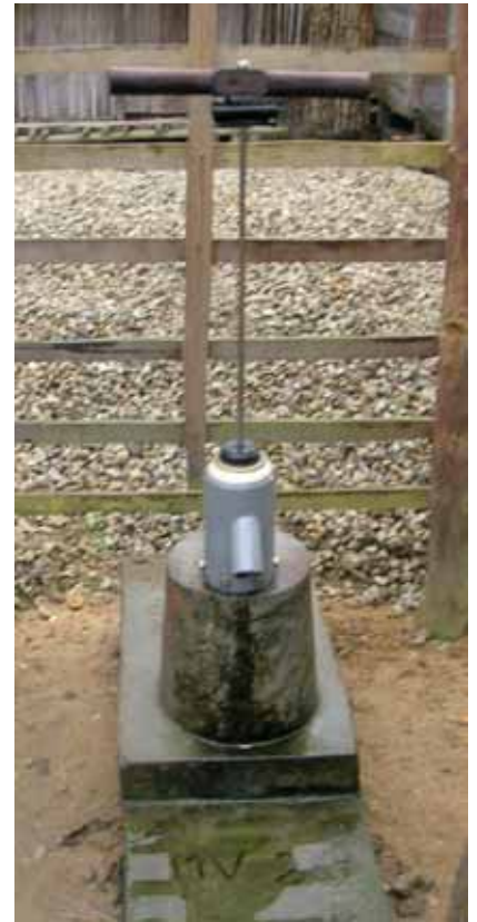
Mahalevona MV 26, hard to pump (pipes are scratching)
