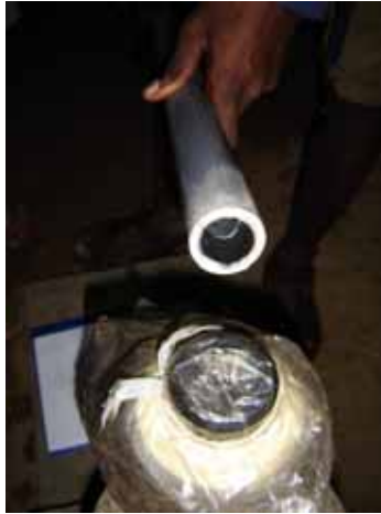
Mahalevona MV 25, slipped pumprod joint
