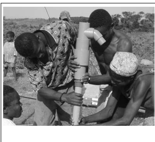
Photograph 2. The pump is installed by the well users themselves.
