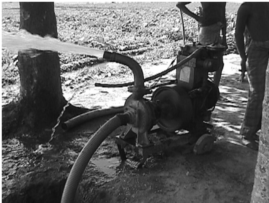
Figure 18: Flow from an Installed 3" Diesel Pump
