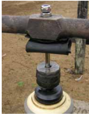
Rantabe R 01, pumprod too long (see additional rubber washers)
