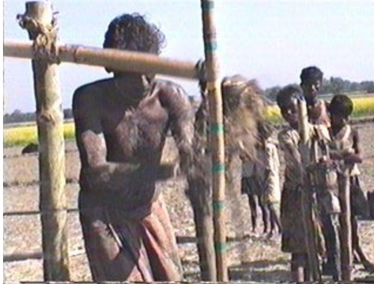
Figure 2: Sludge Ejecting from the Pipe
