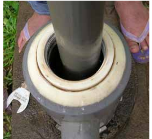
Andranofotsy AB 04, eccentricity, (sign of a bent rising main)
