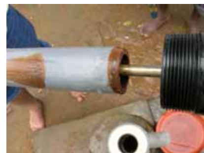
Pumprod pipe edge with wearing marks
