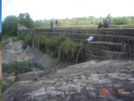
Picture 8. Leakage through masonry section of Gumbalo Dam
