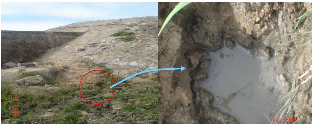
Picture 1 and 2. Leakage at Shagwe dam training wall
