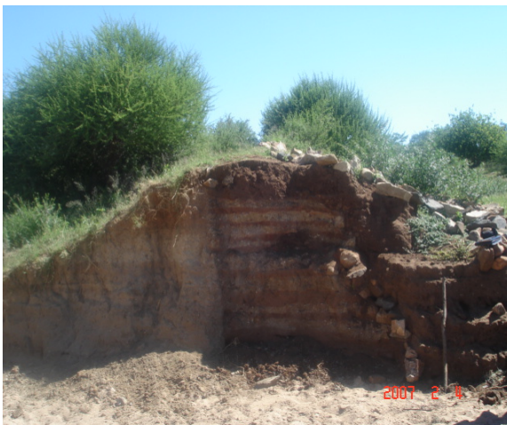
Picture 11. Breached Chobukwa dam wall
