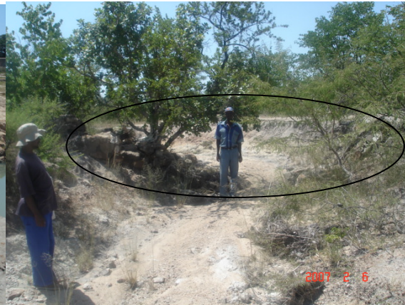
Picture 10. Breached Ngwabi dam spillway sill (Area circled)
