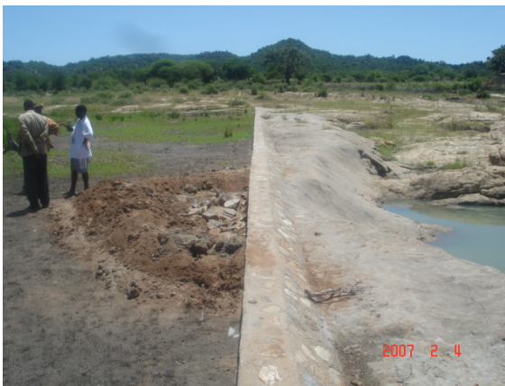
Picture 9. A sinkhole through Makoshe dam spillway sill
