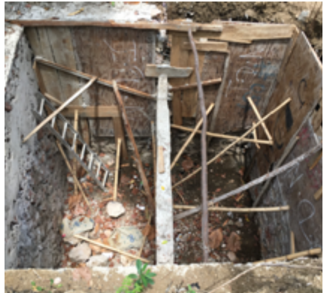
Figure 9. New construction of two-compartment pit for a health clinic, commonly referred to as septic tank in Cap-Haïtien. Photo credit: Anthony Kilbride
