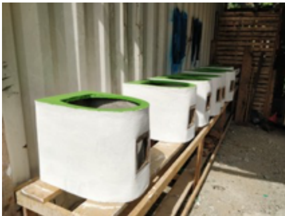
Figure 13. Construction of SOIL CBS toilets using locally available materials (concrete). Photo credit: SOIL
